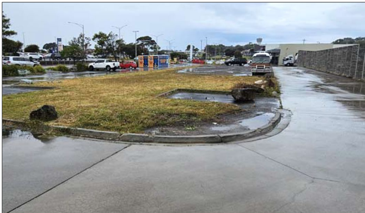
Figure 6.3 Northwest Corner of Site with Wheel Tracks Over Corner of Kerb
