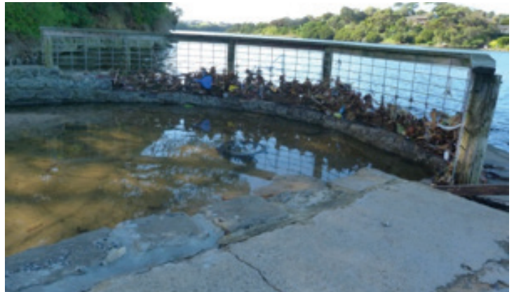
Above: pipe and mesh outfall net. Small items, including cigarette butts still pass through and enter the Hopkins River.
